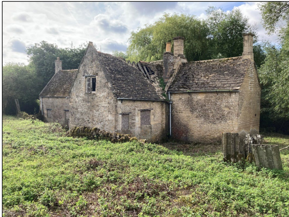
Figure 10 The house from the north-west looking south east. The retaining wall runs across the picture; behind it the ground drops c.1.5m.
