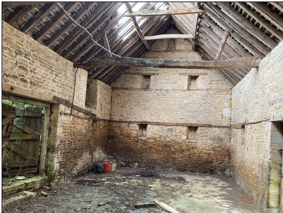
Figure 16 The barn interior, east end. The barn is probably 18 th -century, but with later reroofing. It has opposed doors in the long walls, and five generous ventilation slits (now blocked) in each gable.
